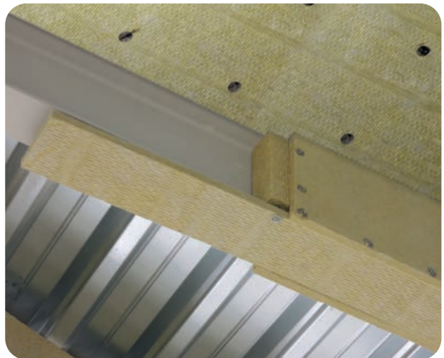
Fig. 16 The three side fire protection of a steel member in combination with the fire protection of a trapezoidal profile sheet. The thickness of the fire protection cladding Isover FireProtect® on the metal sheet corresponds to:
